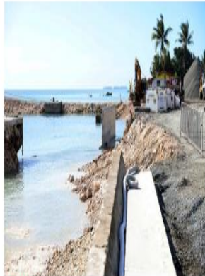
Shoring up: A sea wall being constructed at the Port of Funafuti in Tuvalu as seen on September 6. REUTERS
