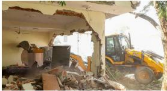
Wheels of injustice: Workers razing the property of an accused in an RSS attack case in Jaipur in October, citing violations. PTI
